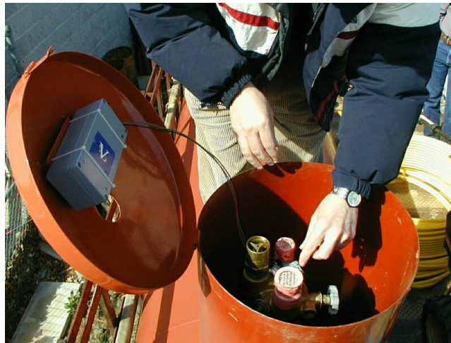
Aprize Tag in Use on LPG Tank
